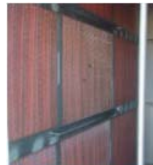
3 of the Style B pre-filters span one inlet hood.
