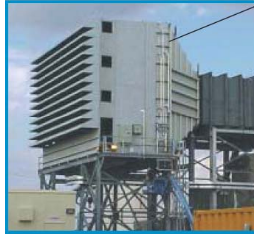
Evaporative cooler section is typically located behind filter section
