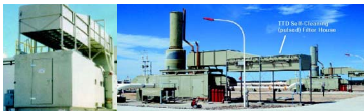
TTD self-cleaning air filter protects a Solar turbine in the hot, arid and dusty environment in Nevada, USA.
